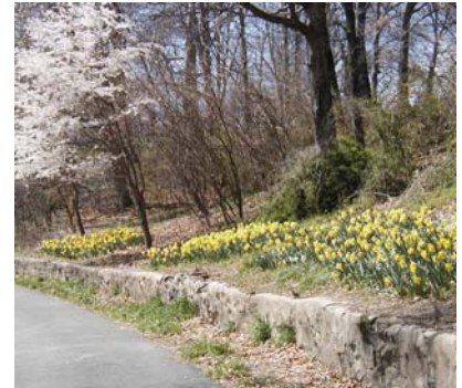
The stone wall is one of the most distinct features but is in poor repair.
